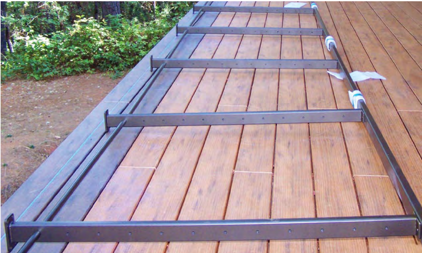
Figure 10: All posts are connect to top rails, spreader bar is installed. Your railing is ready to bring upright.
